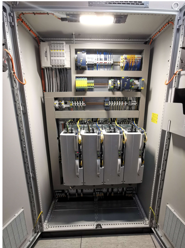
Azimuth Control Cabinet
