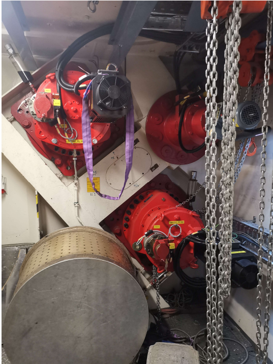
Left Elevation Motors
