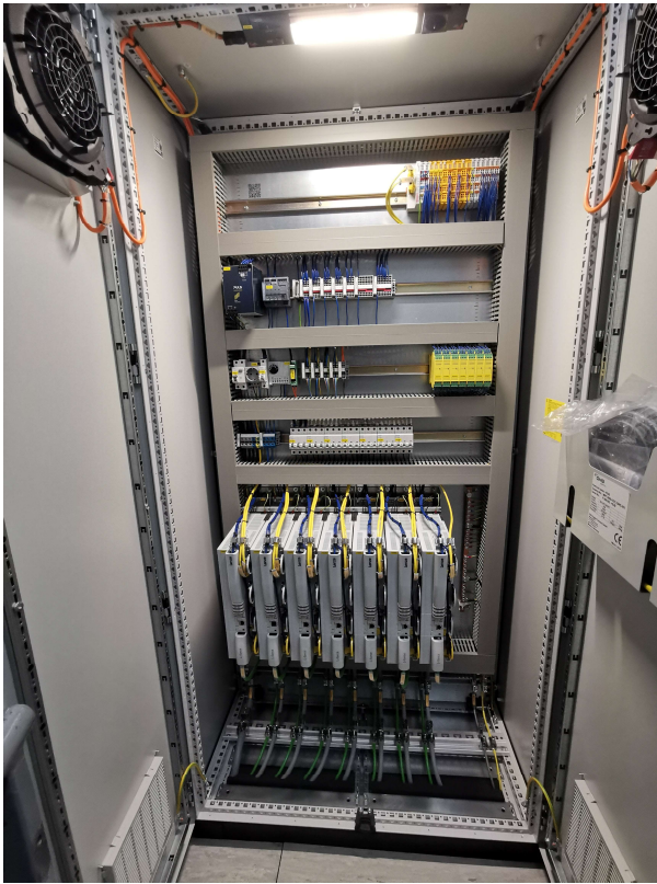
Hexapod/subreflector Control Cabinet
