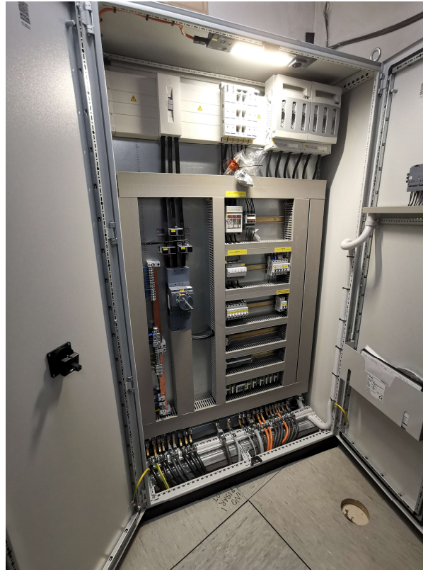
Power Control Cabinet
