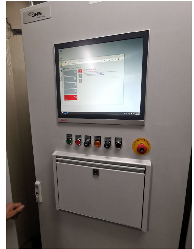
Main Control Cabinet
